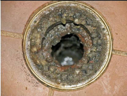
Typical moth fly infested floor drain – Photo by Jeff Tucker
